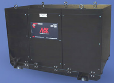
LFP BATTERY BANK
